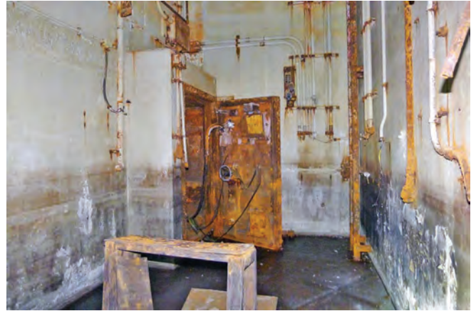
The interior of the personnel blast-block with a very rusty blast door
